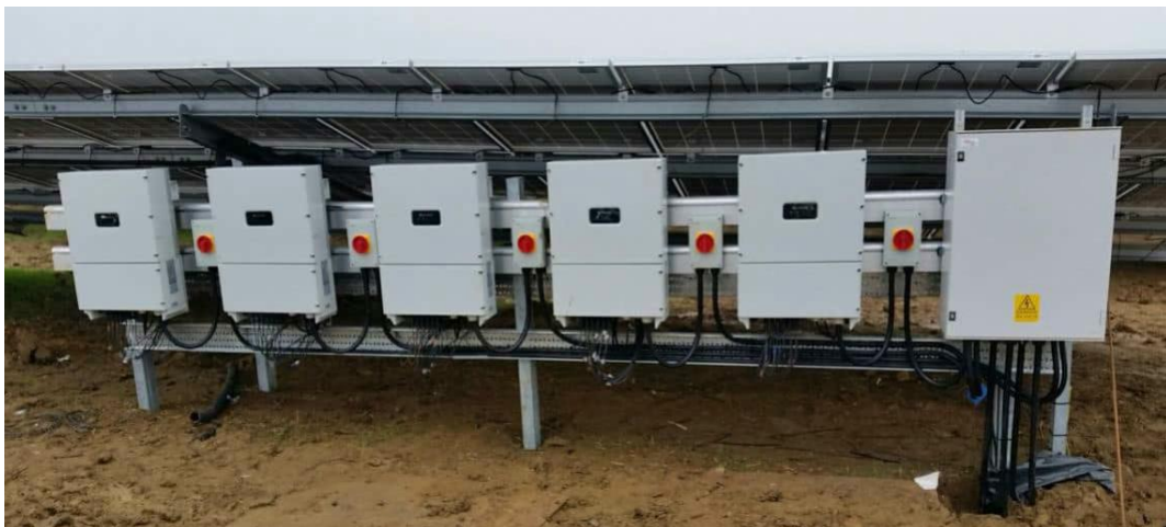
Plate 3: Typical String Inverter Installed Next to Solar PV Panels
