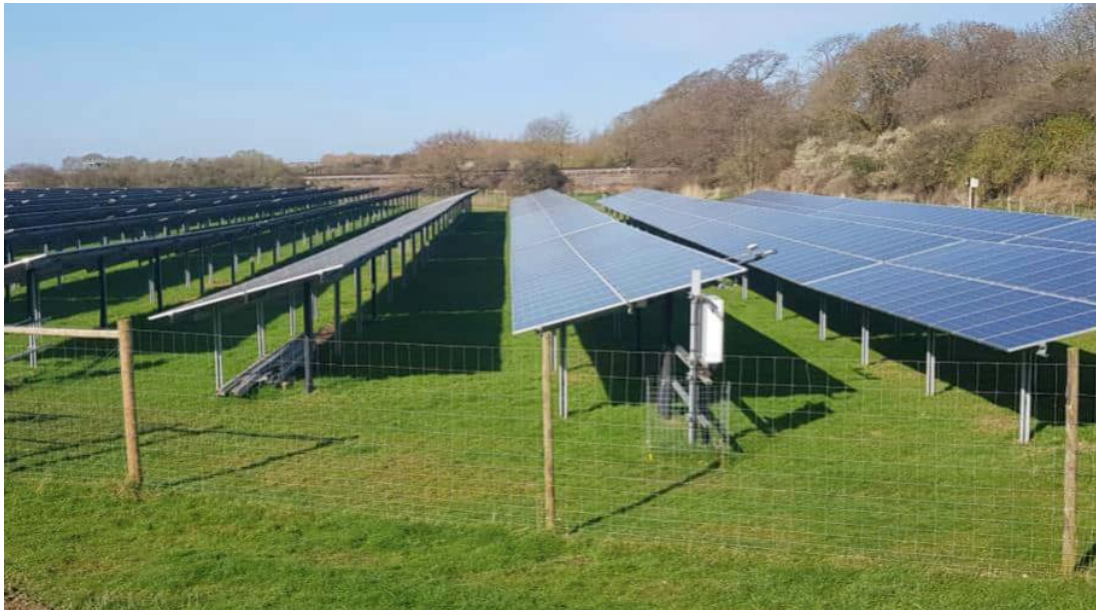
Plate 2: Example South Facing Solar PV Panels
